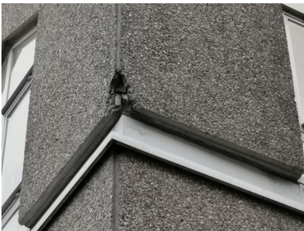
Plate 8: showing damaged rendering
