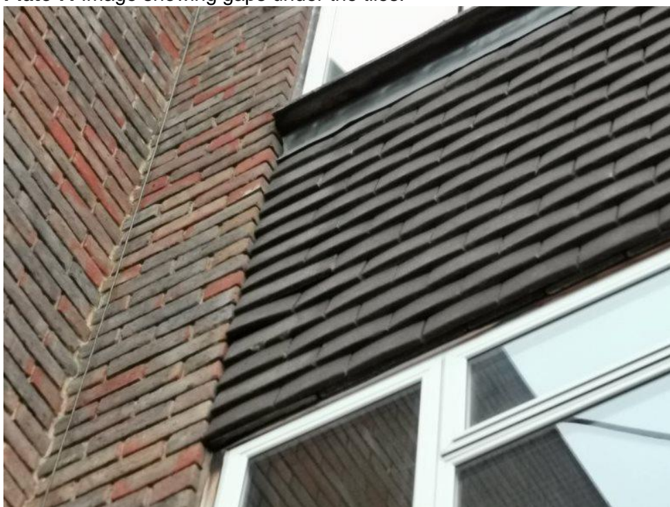
Plate 7: Image showing gaps under the tiles.
