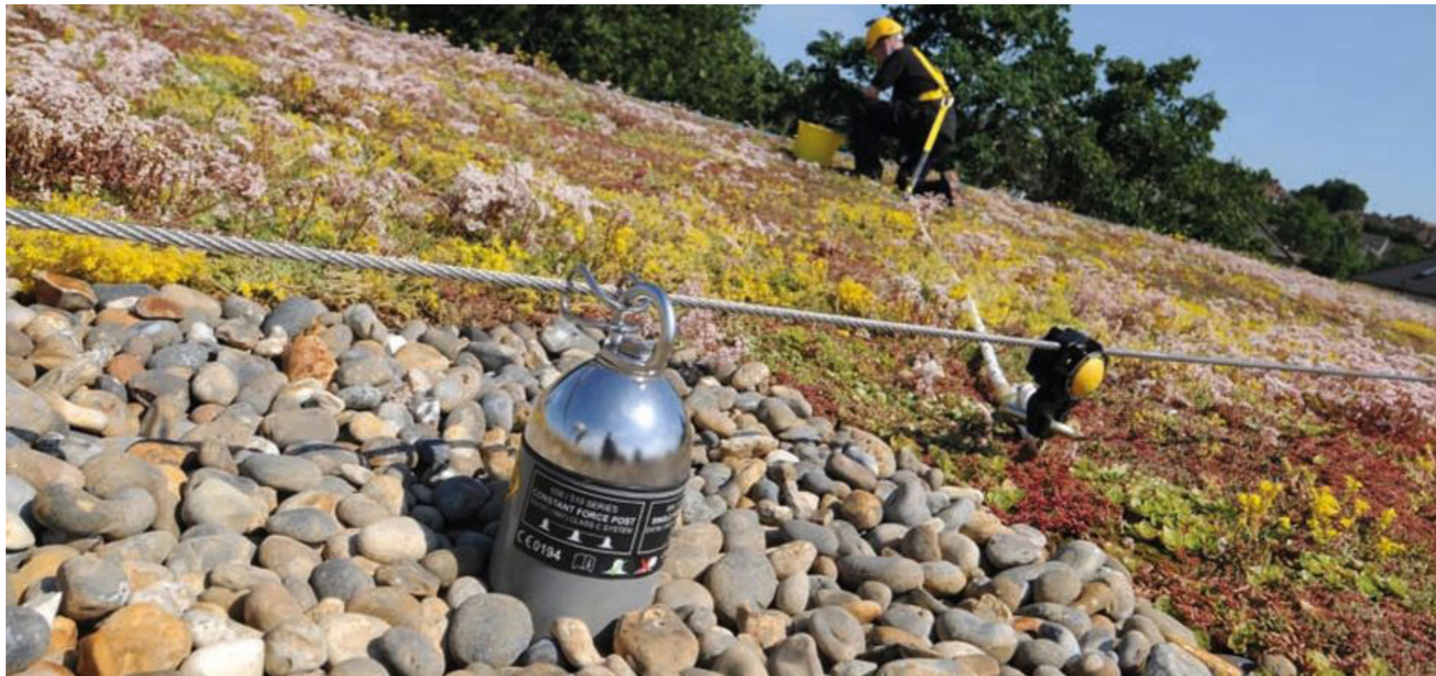
01 Mansafe system to green roof
