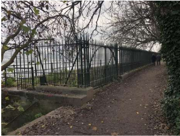
End of wharf where water and electrical connection points are located. Foliage can be seen in the wharf wall.
