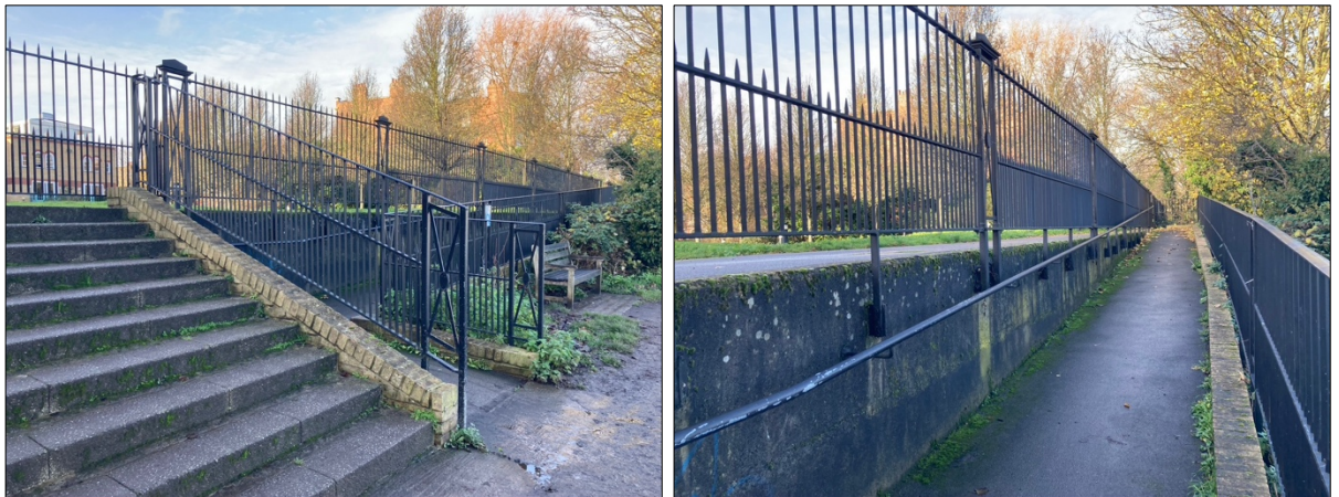
Photograph 5a & b. A view of the existing access ramp and steps, north of the wharf.
