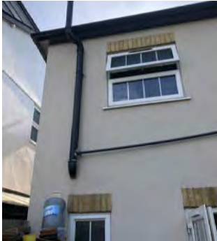
UPVC windows, downpipes and soil pipes
