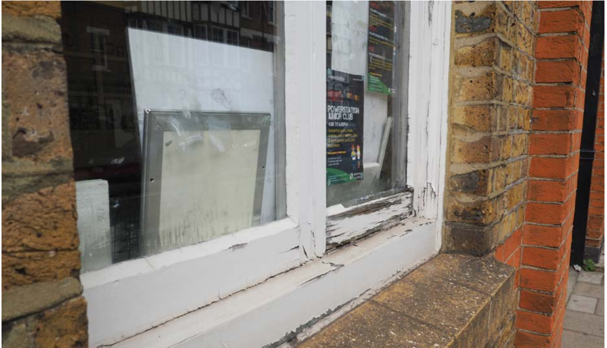
Detail showing deterioration of fenestration
