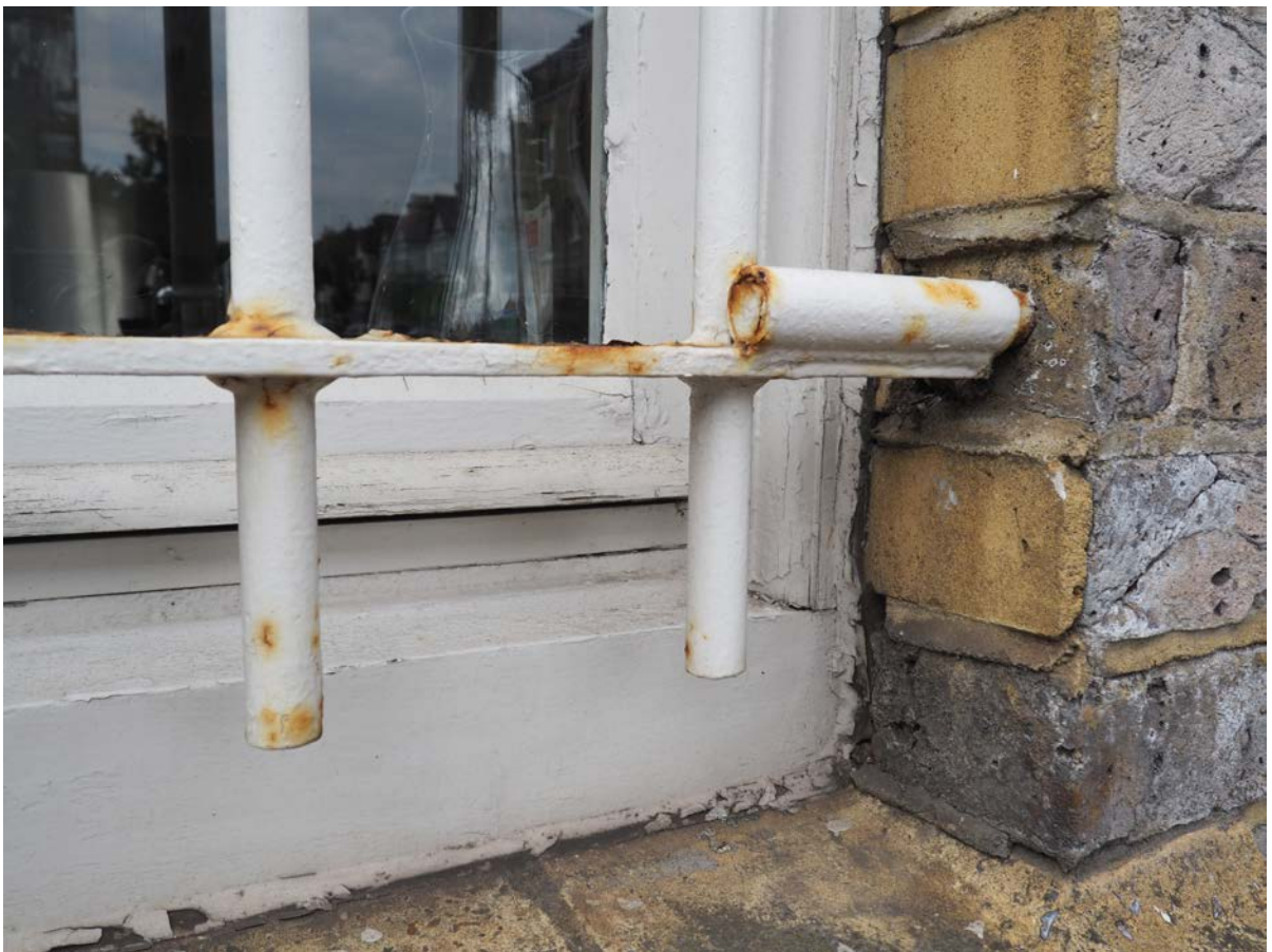
Detail including security bars to be removed
