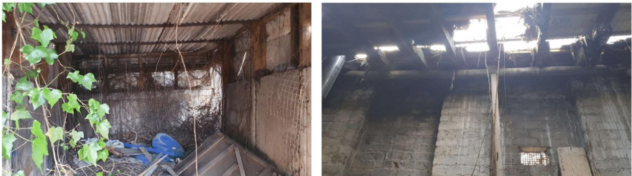
Figure 7-1 - Images from Building Survey Report showing poor condition of outbuildings.
