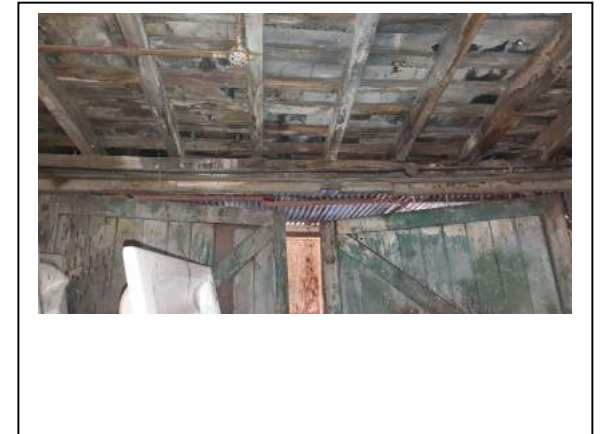
27. Failure of roof structure
