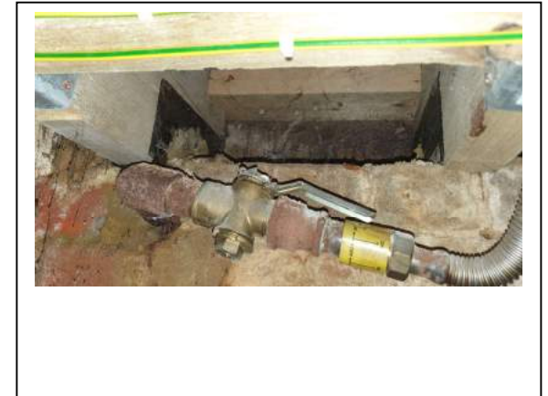
57. Gas valve basement no 31
