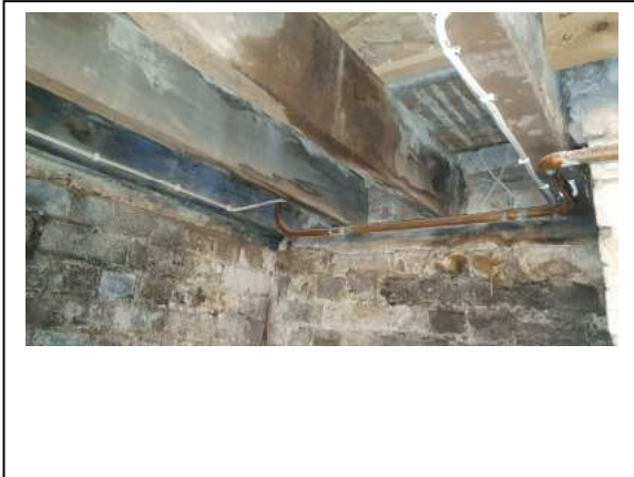
58. Water damage to ground structure no 31
