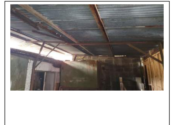
24. Failed structural members
