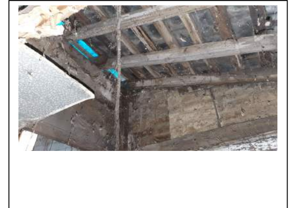
30. General poor condition of structure
