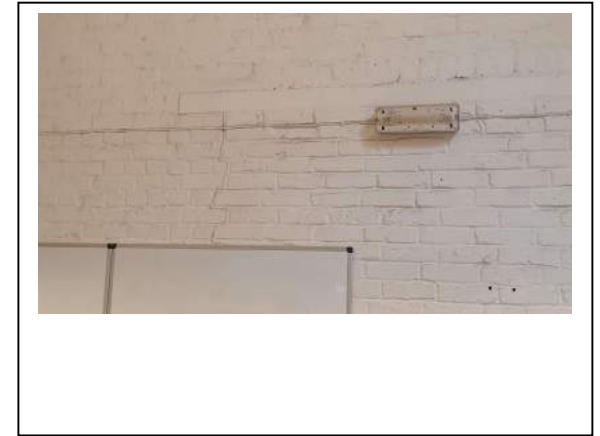
51. North wall 1 st floor cracking
