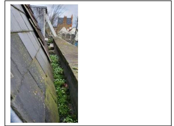
21. Hidden gutter to High St of 31
