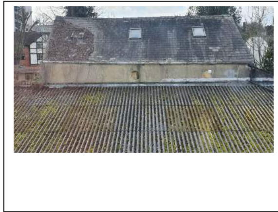
20. Asbestos sheet roof, damaged elevation and slate roof overloading roof
