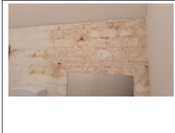
53. Water damaged internal wall 1 st floor east elevation
