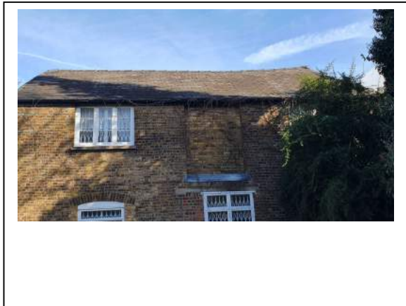
10. Bowing roof of 29B
