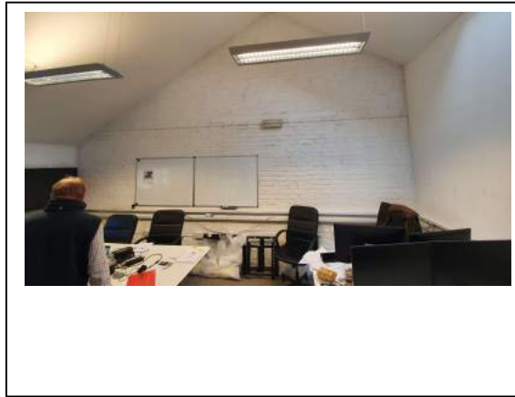
50. North wall 1 st floor cracking through
