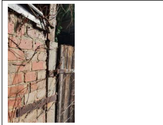
35. Movement in wall and entrance
