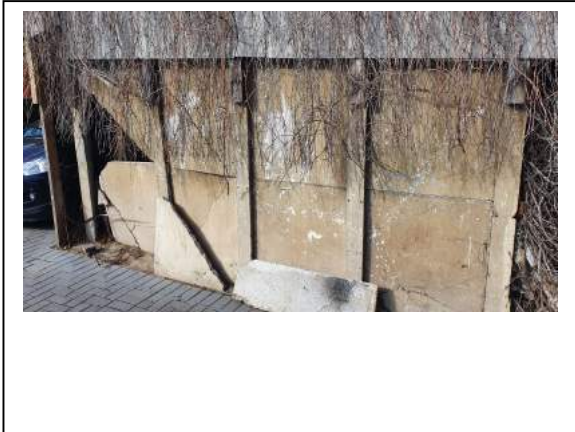
34. Failing elevation / structure
