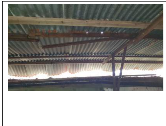
23. Failed structural members
