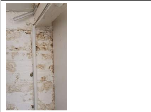
52. Water damaged internal wall 1 st floor east elevation
