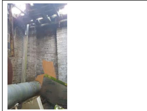
29. Poor structure and roof covering
