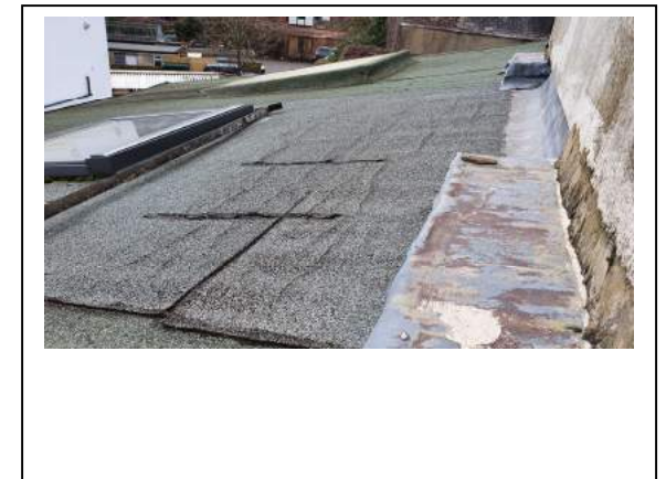
18. Poor felt roof covering to no 29 1 st floor
