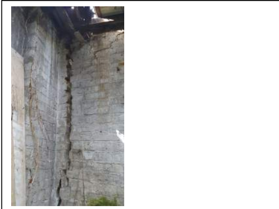
28. Significant cracking to rear / flank wall
