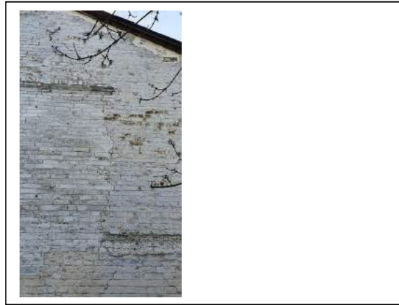
8. Cracking to elevation
