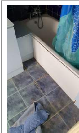
61. Poor bathroom tiling
