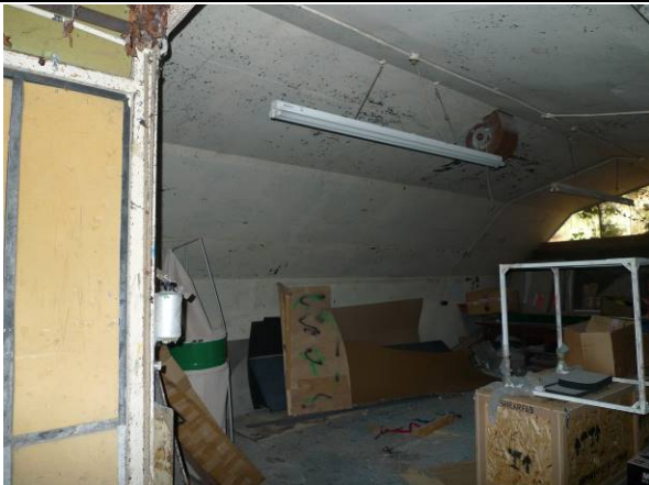
Photo 15 – Building B7 showing the boarded out roof and the clear windows on the eastern elevation.
