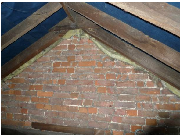
Photo 11 – Southeastern gable showing gaps stuffed with insulation and the poor state of repair of the brickwork.
