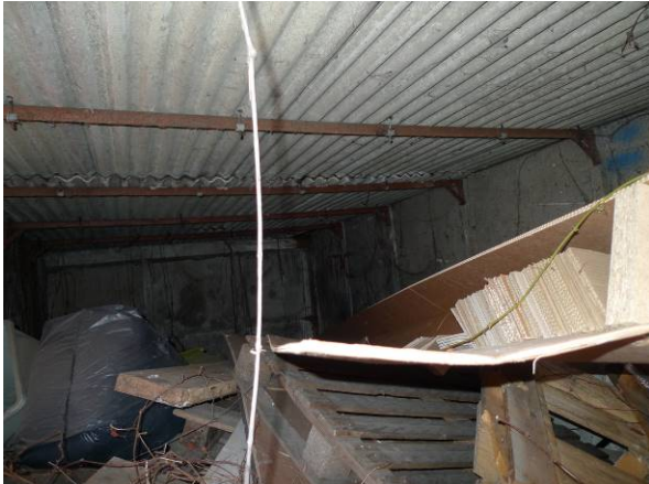
Photo 13 – Building B5, a single storey dilapidated garage with asbestos corrugated roof and missing side panels.
