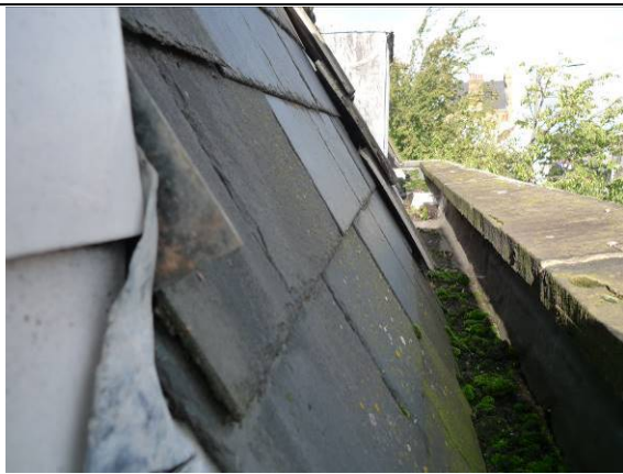
Photo 9 – Gaps around the lead flashing and between the slate roof on site and the tiles of the neighbouring property.
