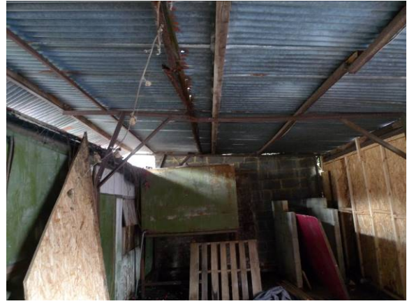
Photo 14 – Building B6 looking west with chipboard frontage and metal corrugated roof with large gaps. The doors to Buildings B8 and B9 are shown on the left of this photograph.
