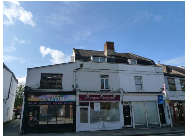
Photo 1 – North-eastern elevation of Building B1 that is adjacent to the High Street. Note the dormer windows in the roof.
