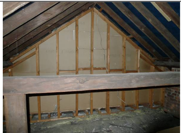
Photo 10 – Roof void of B1 showing an open uncluttered space and the partition wall for the neighbouring building.
