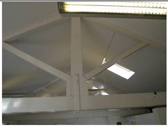
Photo 12 – Roof of building B4 showing the lack of an enclosed roof space.
