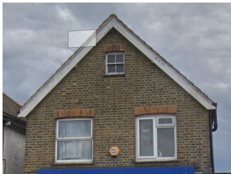
Soldier brick course above windows and at floor slab levels on neighbouring buildings.
