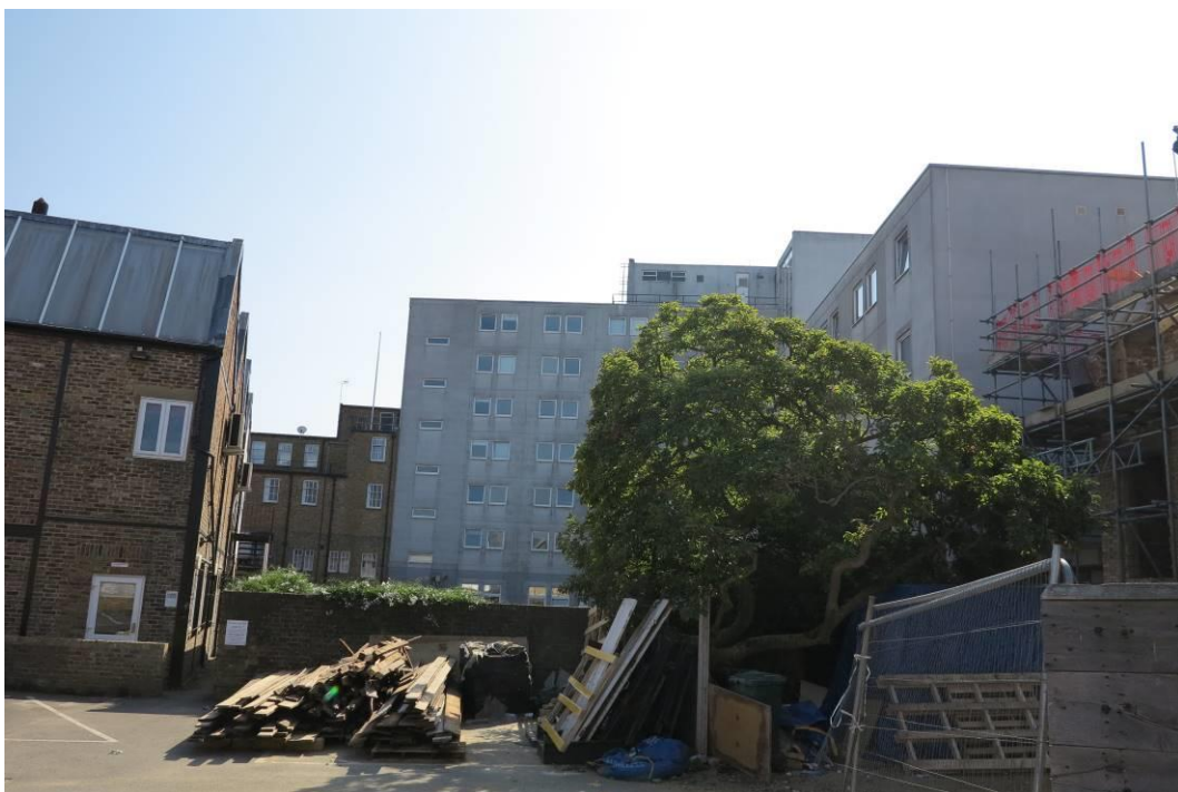
Plate 22. View towards Kingston Bridge House from the car park to the rear of 4 Church Grove
