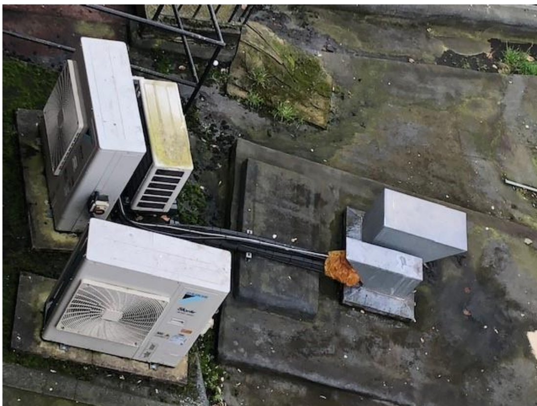
Figure 5: Plant on Neighbouring Lower Roof
