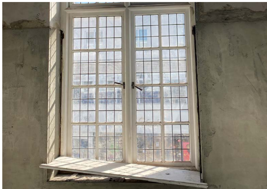
Figure 4.10 Bottom half of an original window on the south-east elevation at first floor level.
