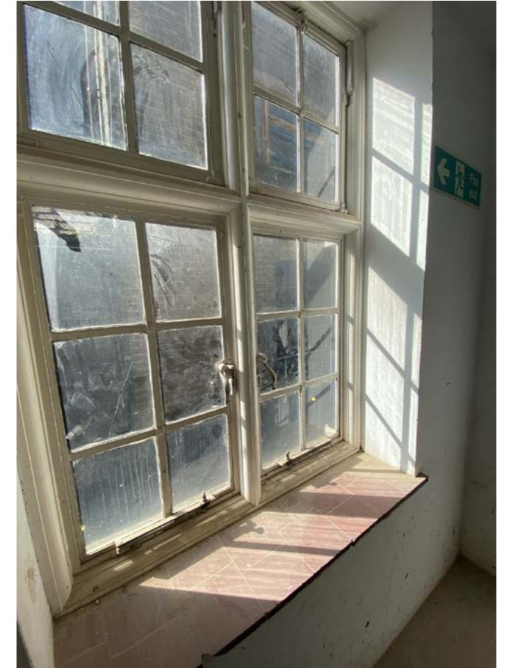
Figure 4.8 Casement window in the stairwell of the north building, inserted sometime after 1928.
