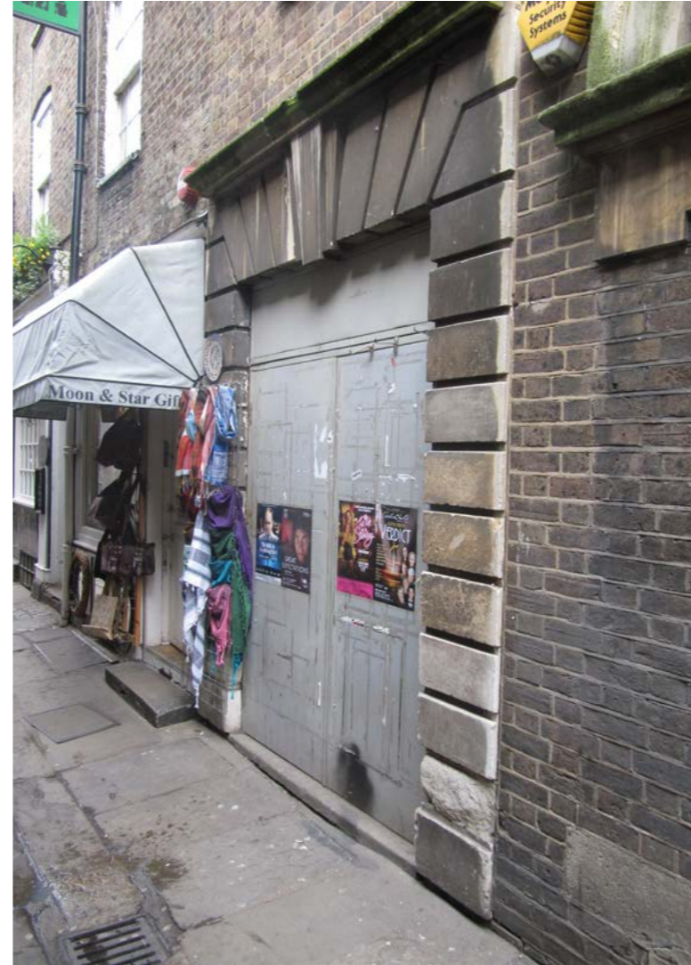
Figure 4.4 Rusticated stone door architrave at ground floor level on the south-west elevation.
