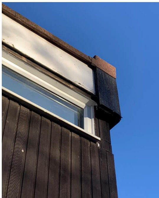
Photograph 9 PRF: Hole in timber sarking (Target note 3)
