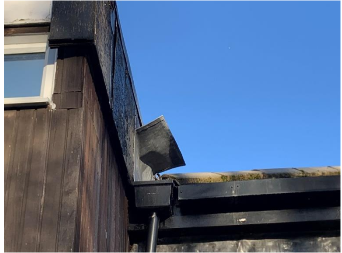
Photograph 4 PRF: Hole in timber sarking
