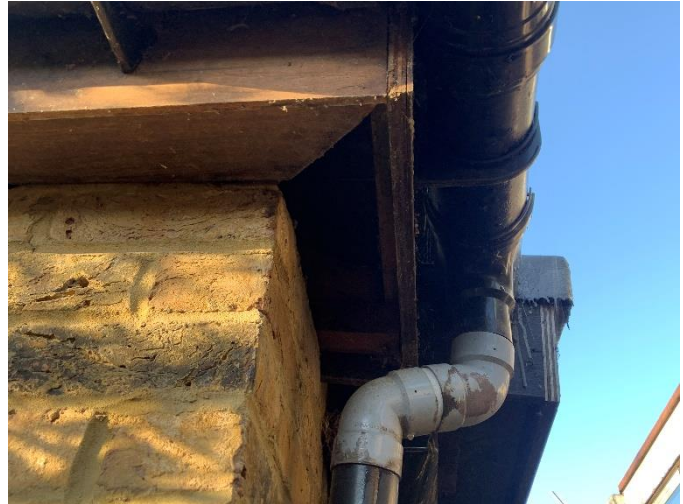
Photograph 5 PRF: Hole in soffit box
