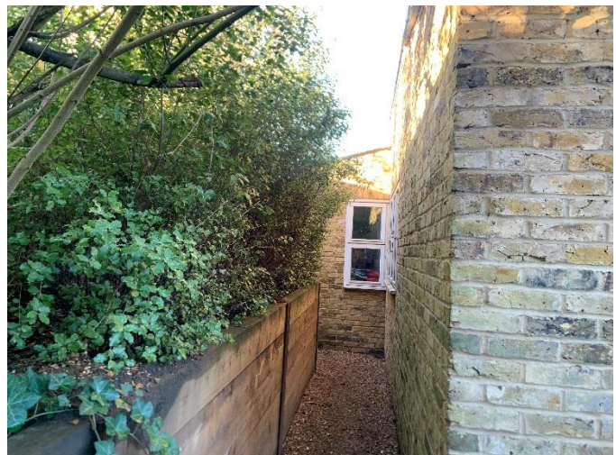
Photograph 6 Eastern elevation of building section B1.8, single storey extension adjacent to B1.2 with no PRF's.
