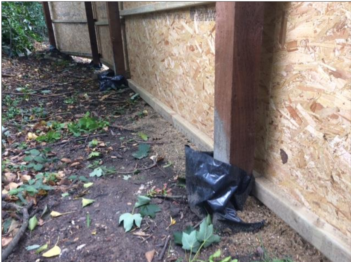
Fig. 3 Liners inserted into the post hole before setting the post in position with concrete
