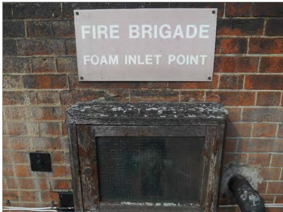
Photo 14: In case of fire facilities
