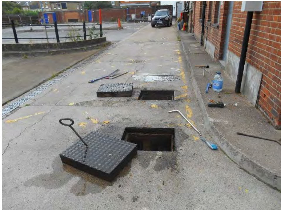
Photo 37: Underground drainage pipes
