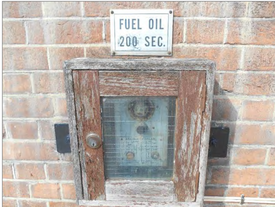
Photo 13: Fuel oil dispenser
