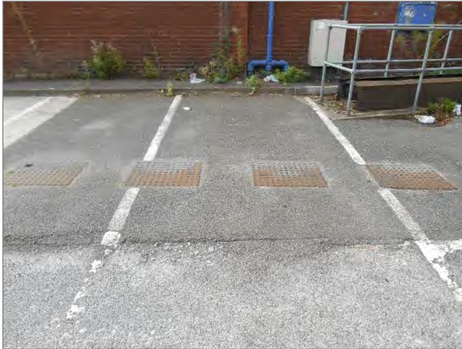
Photo 7: Interceptor tank located at the front of the station
