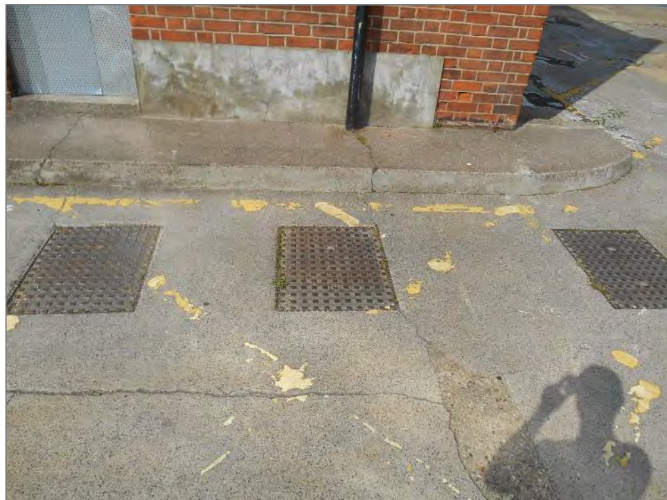
Photo 18: Underground drainage pipes
