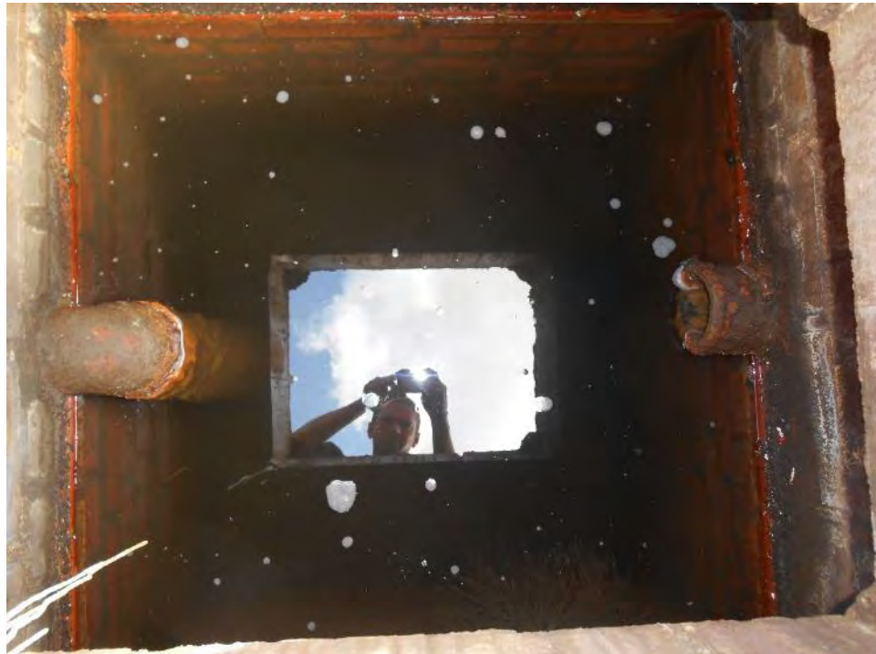
Photo 33: Conditions inside the interceptor
