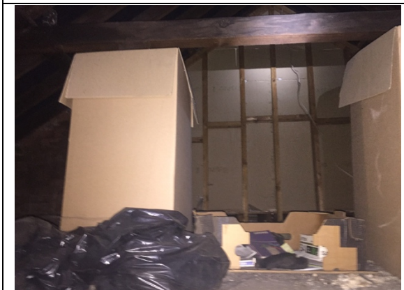
Photo 5: Roof void of B1 showing an open uncluttered space and the partition wall for the neighbouring building.
