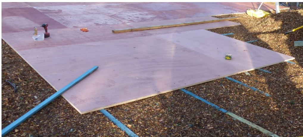
Fig.1 Ply-boards placed onto a layer of woodchips provides a good working surface for pedestrians or scaffolding
