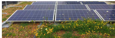
Fig. 3 & 4 PV Panels mounted on green flat roof
