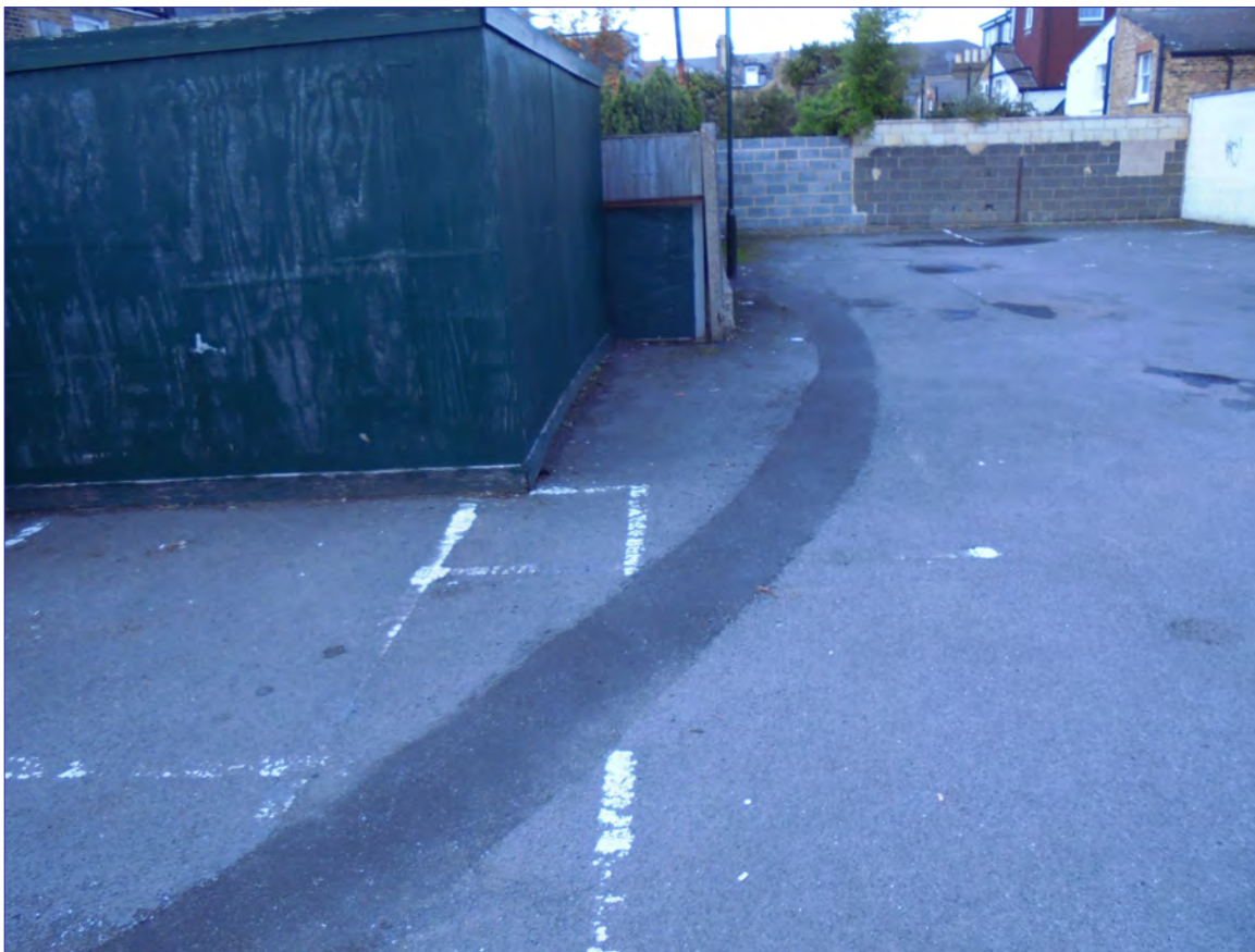
Plate 6: Detail of cable trench disturbance in the northern part of the Site
