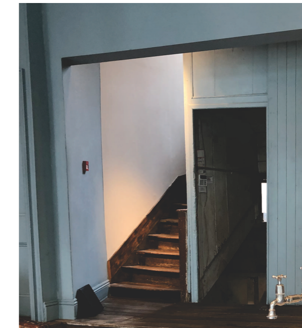
VIEW 1 NEW 60MIN FIRE RATED PARTITION TOP TO BE INSTALLED ACROSS EXISTING OPENING AT FOOT OF STAIRS
