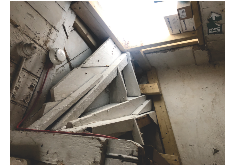
VIEW 3 UNDERSIDE OF EXISTING STAIRS TO BE CLAD IN PLASTERBOARD TO ACHIEVE 60 MIN FIRE PROTECTION
