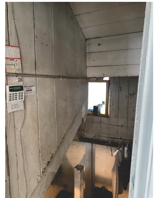
VIEW 2 EXISTING STAIR PANEL TO BE CLAD IN PLASTERBOARD TO ACHIEVE 60 MIN FIRE PROTECTION
