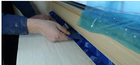
The image above shows an example window frame being taped to a masonry wall before the sill and window reveal are installed.
