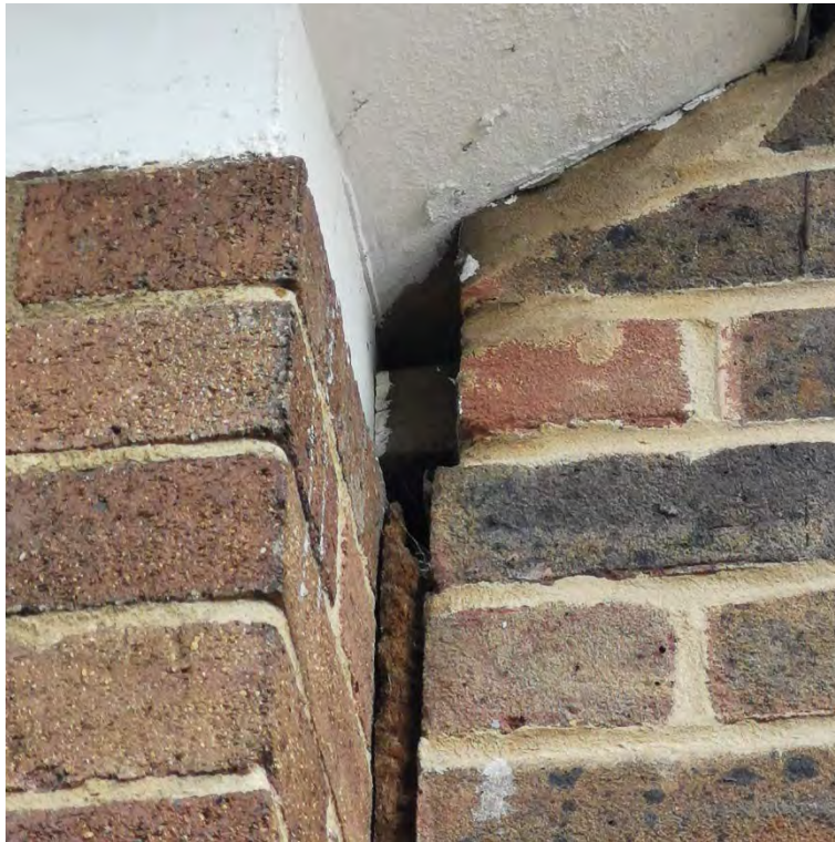
Photograph 25 – Missing mortar at join of B6
