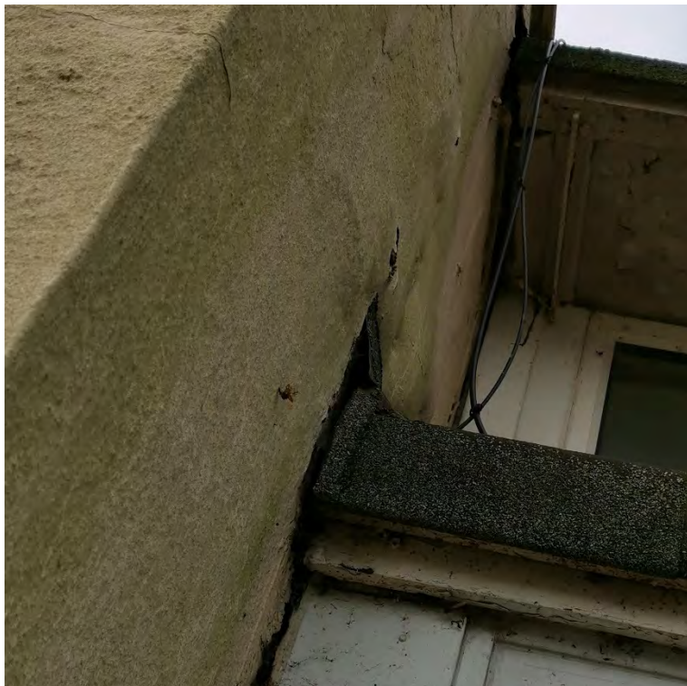
Photograph 12 – Gap between felt and wall on B2
