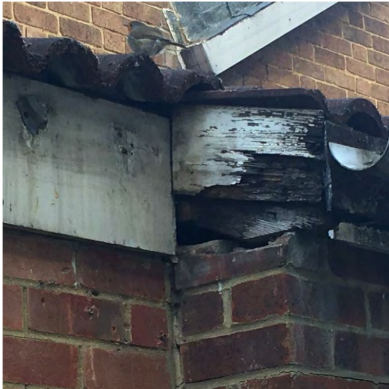
Photograph 32 – Rotten soffit on B9
