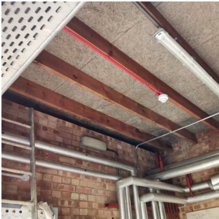
Photograph 18 – Gap above wall in boiler room associated with B3
