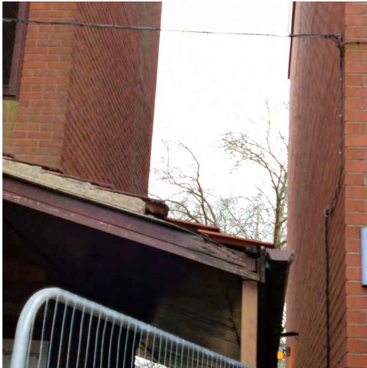
Photograph 17 – Rotten fascia forming gap under tiles on porch of B3
