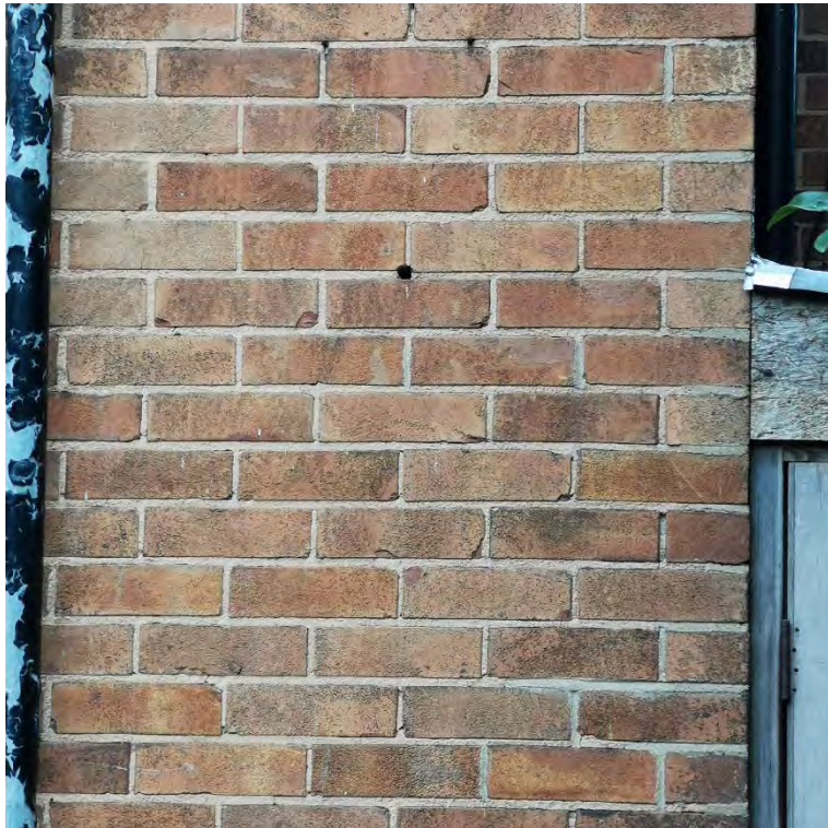
Photograph 22 – Hole in brickwork on B5
