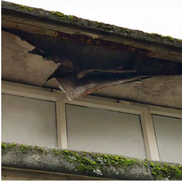
Photograph 13 – Torn soffit on B2
