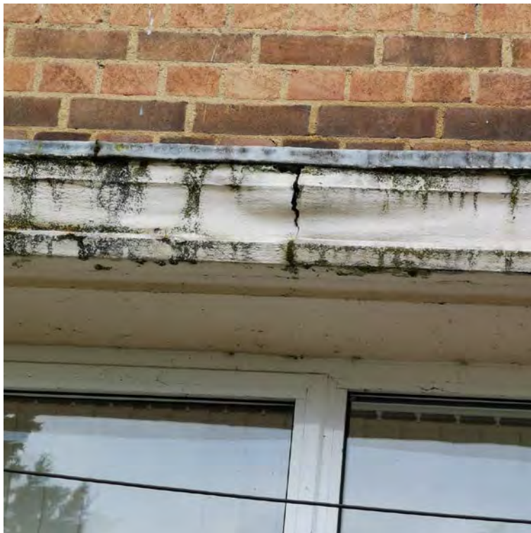
Photograph 16 – Crack in stonework on B3
