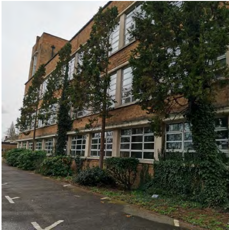
Photograph 1 – Lawsons Cypress trees to west of B3, Tree 3 and 4 are ivy clad
