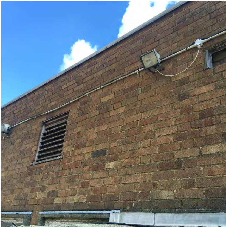
Photograph 31 – Vents and gaps in brickwork on B9
