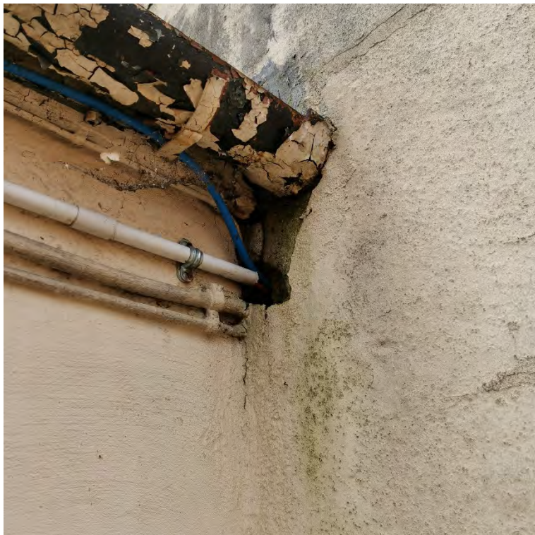
Photograph 8 – Hole on north-eastern aspect of B1
