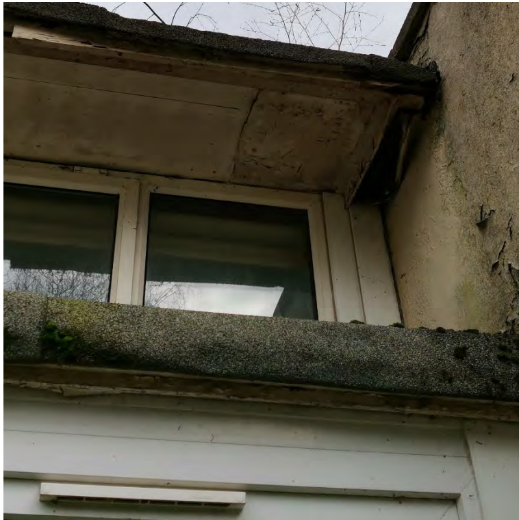
Photograph 9 – Rotten soffit on south-western aspect of B1
