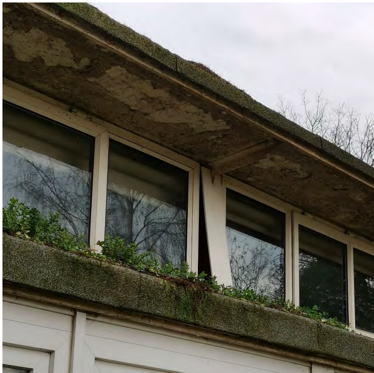
Photograph 10 – Lifted panel between windows on B1
