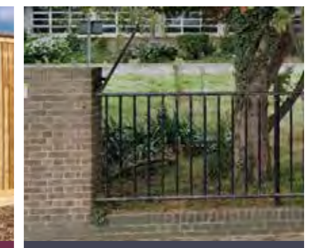
Boundary type 7 - Egerton Road Refurbished brick wall upstand with metal railing topper (height as existing)
