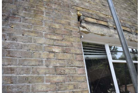
Figure 9: Absence of Lintels to Support Brick Work
