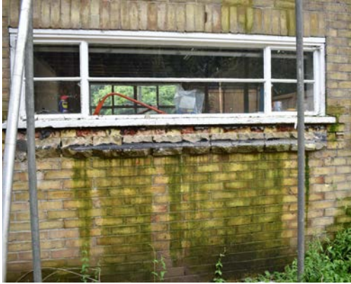
Figure 8: Corroding Metal Windows
