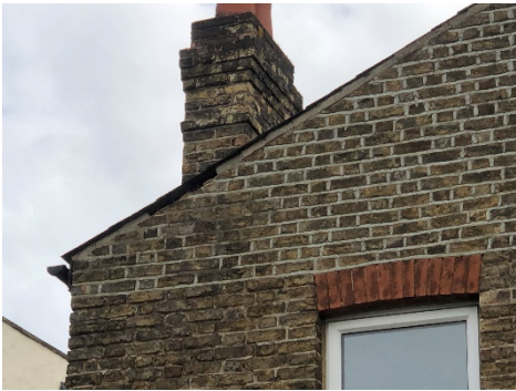
P17: Zoomed-in view of the gap in the building eaves of BN5
