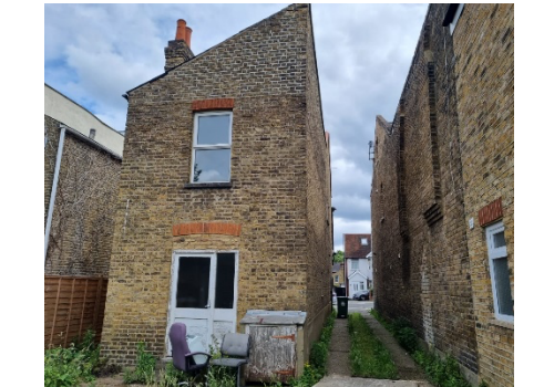
P16: Gap in the building eaves of BN5 and habitats of entrance driveway
