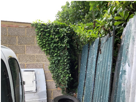
P13: Ivy growth on north- and west-facing walls of BN2
