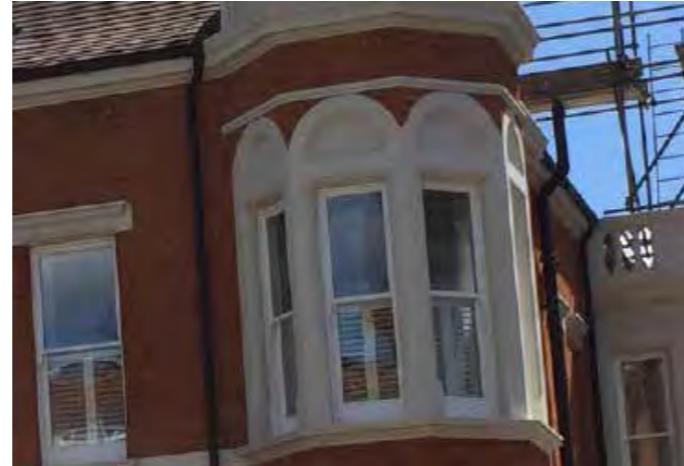
Timber sashes in a Victorian turret
