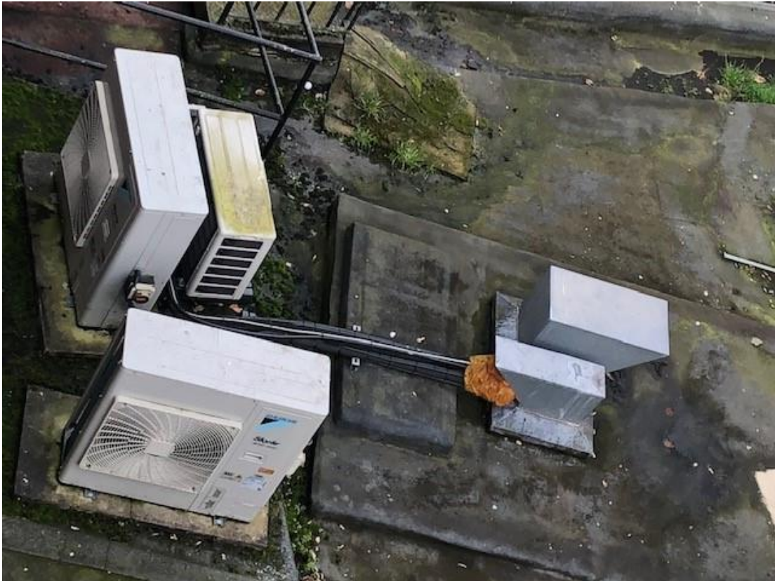
Figure 5: Plant on Neighbouring Lower Roof
