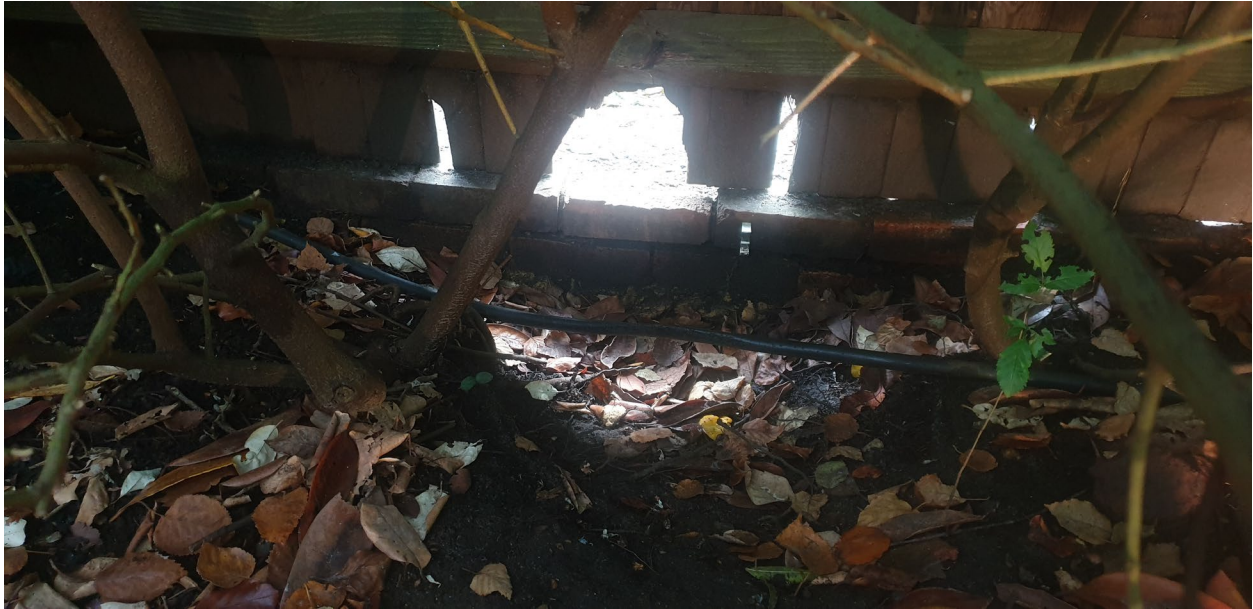
Figure 5: gap beneath southern boundary
