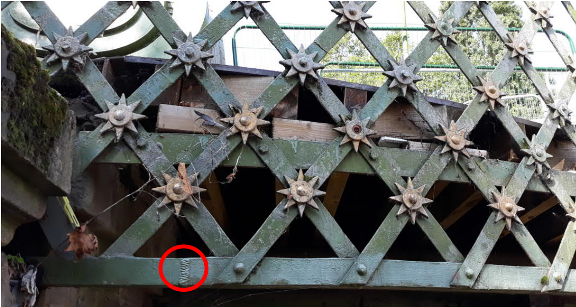
Photo 3.7: Signs of previous cutting and welding of parapet bottom horizontal member (east side of the bridge, near Barnes end abutment)
