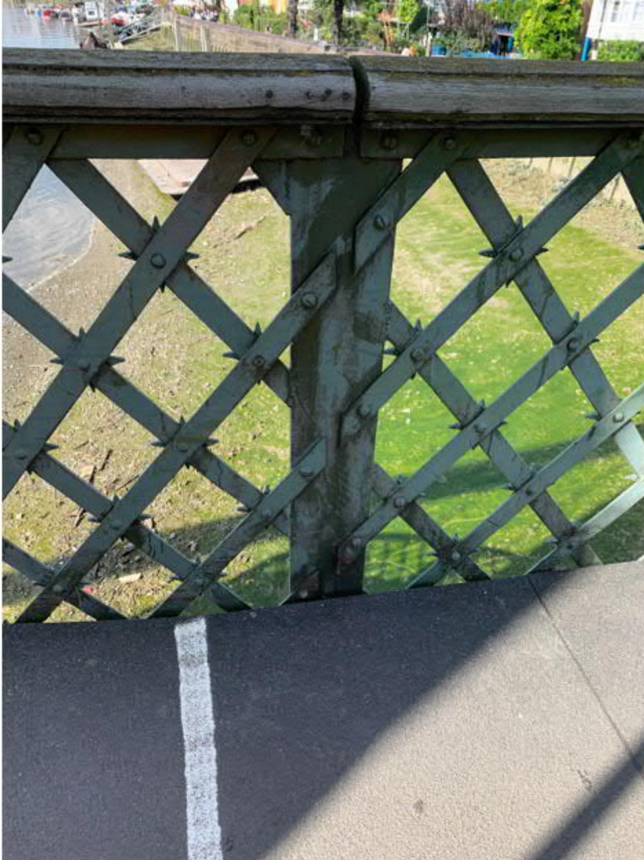
Photo 3.6: Evidence of previous cutting of parapet diagonal members
