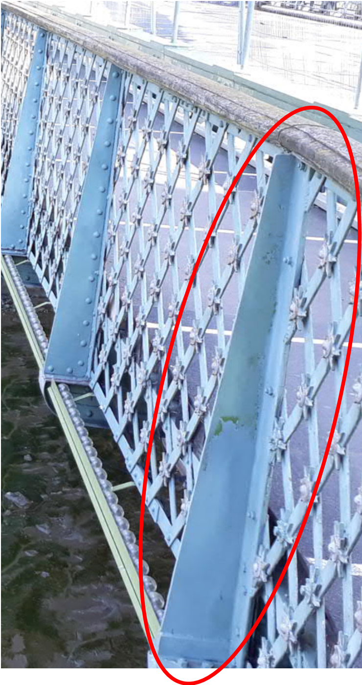
Photo 3.5: Replacement parapet vertical member from previous interventions (west side of the bridge, near the Hammersmith end tower)
