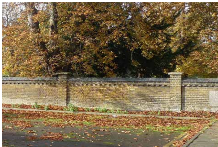
Figure 3.22 The boundary wall between the Site and the Old Mortlake Burial Ground. The wall is broken down in places and in a low to poor overall condition.
