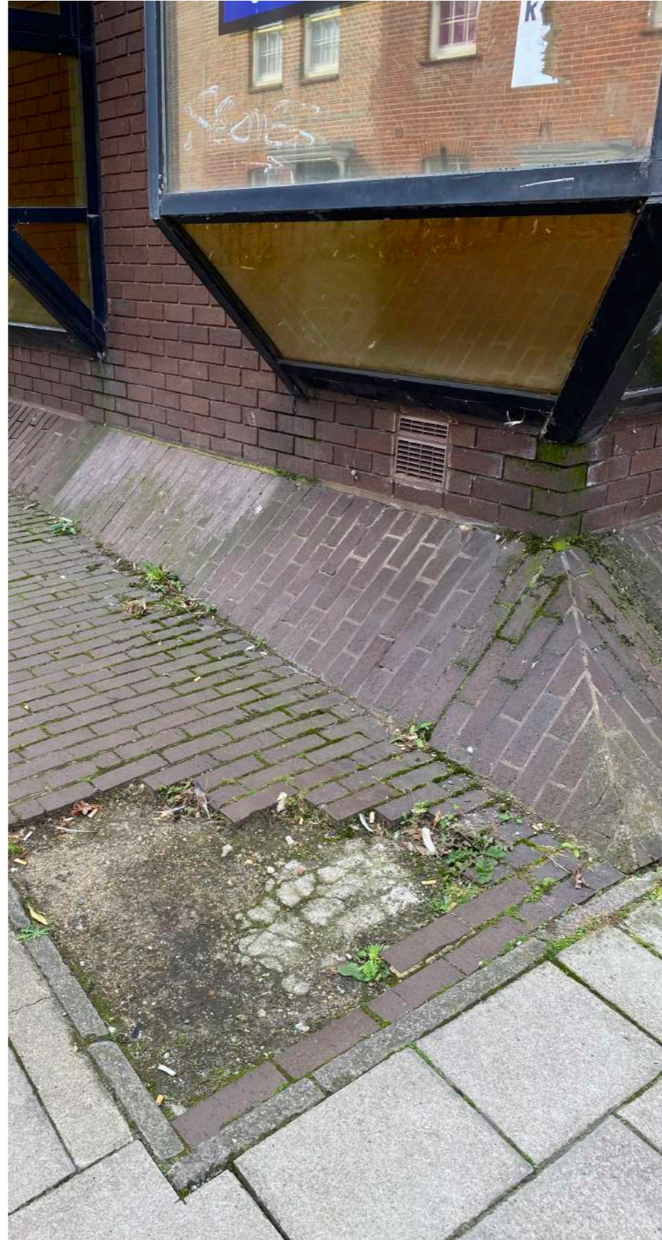
4. Missing Pavers in Public Realm
