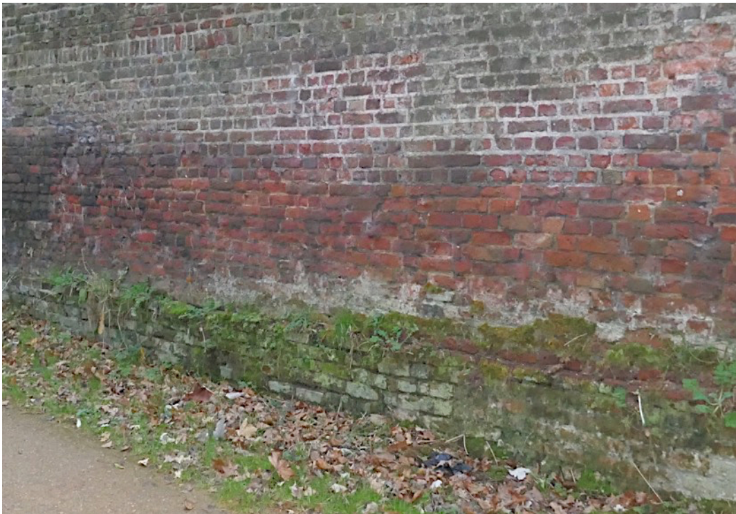
Figure 2;-The mortar bedding in the plinth is completely degraded. The bricks are generally loose but are bound in place by roots and friction.
