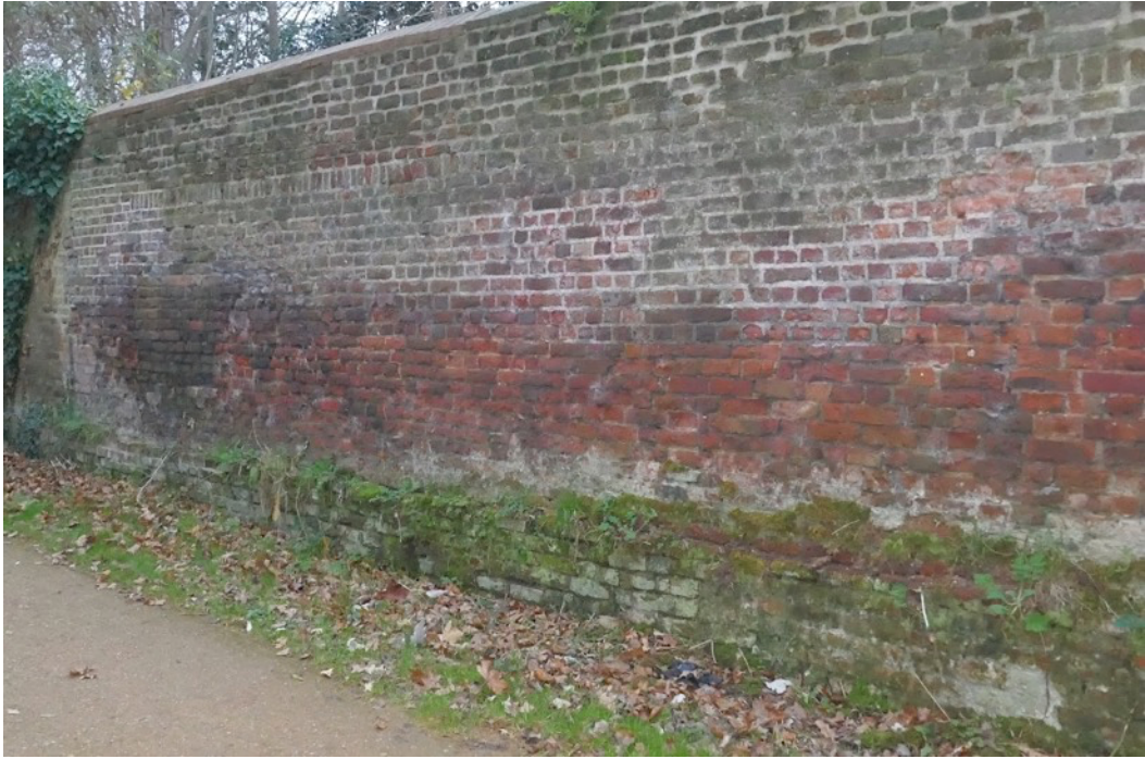
Figure 4;- Another example of brickwork failure in the plinth where the brick remain in place held by the plant roots.
