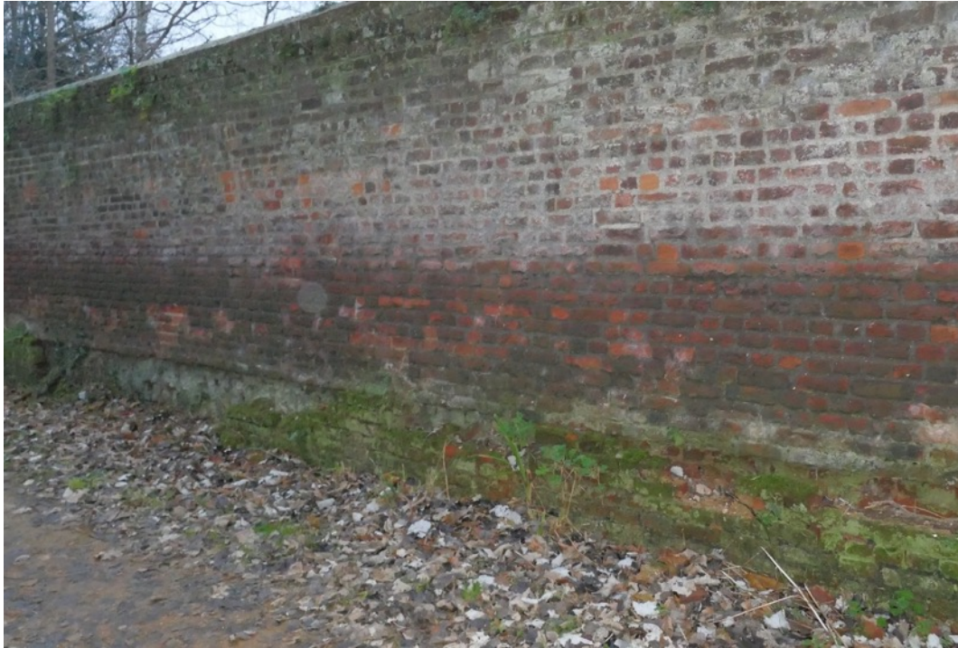
Figure 5;- The plinth has completely fallen away on the left of the picture. The expose core of the wall is heavily colonised with green algae.
