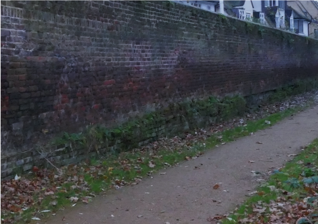
Figure 3;-The bricks in the near plinth are loose as in the previous picture. Further to the right the plinth has fallen away.
