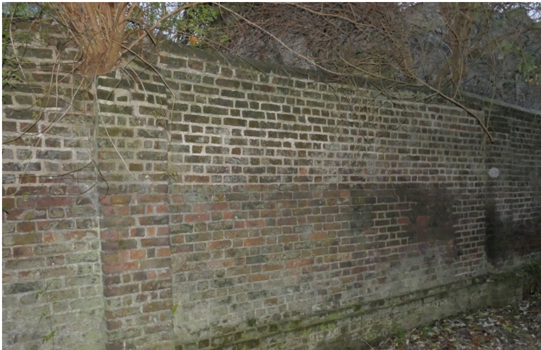
Figure 6;- Embedded semi-mature buddleia plants in top of the wall above the piers have cracked and loosened the brickwork in the wallhead.
