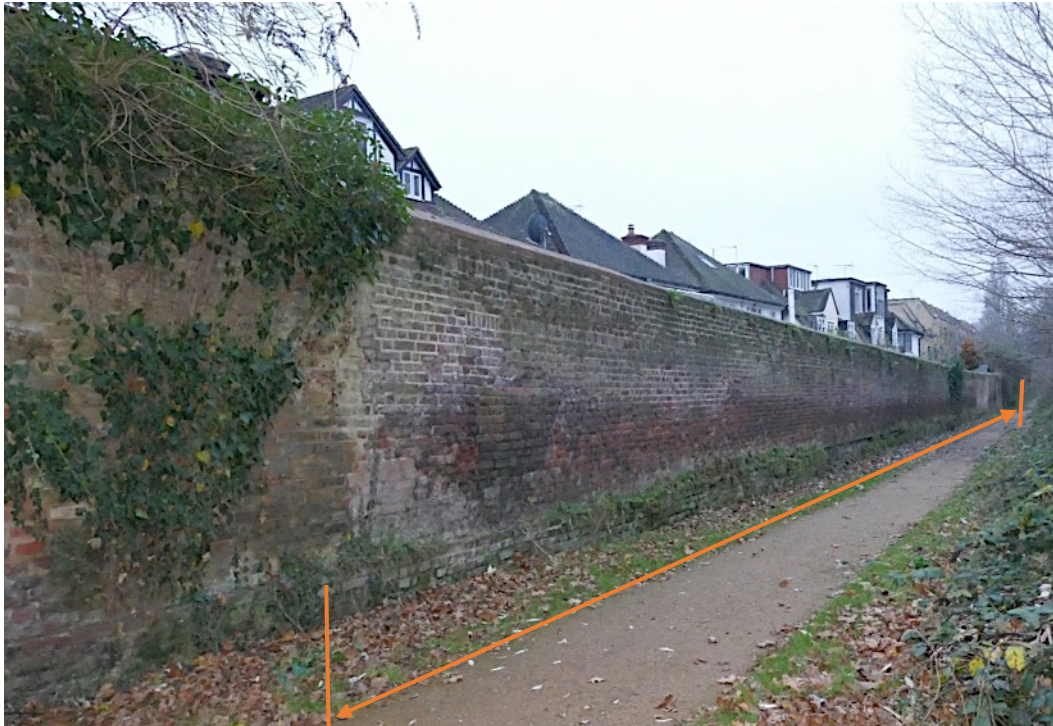
Figure 1:- General view of the area of wall and plinth scheduled for repairs indicated by orange arrows.
