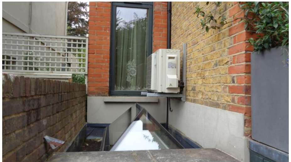
Current position of Unit #6 at ground level. This unit is to be re-located onto the balcony at 1 st floor level.
