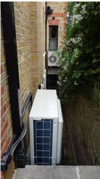
View of Unit #4 in foreground at basement level with obsolete unit #5 in background
