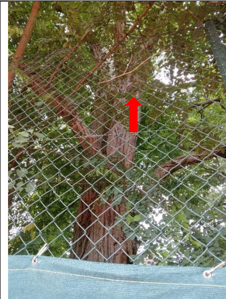
Photograph 3 – South aspect of T1. The location of the branch wound hole is denoted by the red arrow.
