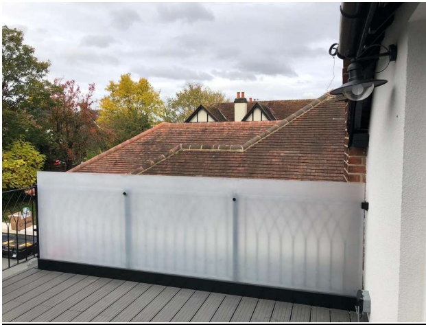
Proposed glazed guard rail previous installation. Our new railing will be transparent glazing.
