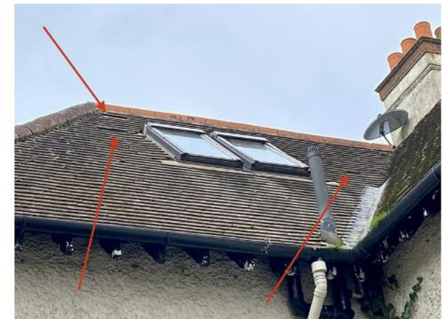
Pictures 9 & 10: Close up images of slipped and raised roof tiles present along B1's western elevation.
