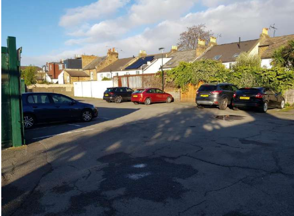
Photo 4: Photo of current condition of asphalt in car park.
