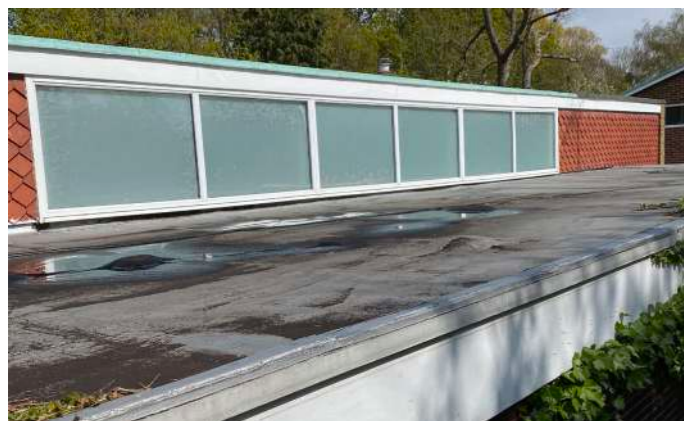
The existing rear clerestory is innovatively redeployed in a set back on the front elevation for north light, and houses a PV array. Overall massing heights are broadly in line with existing, as the red line overlay opposite shows.
