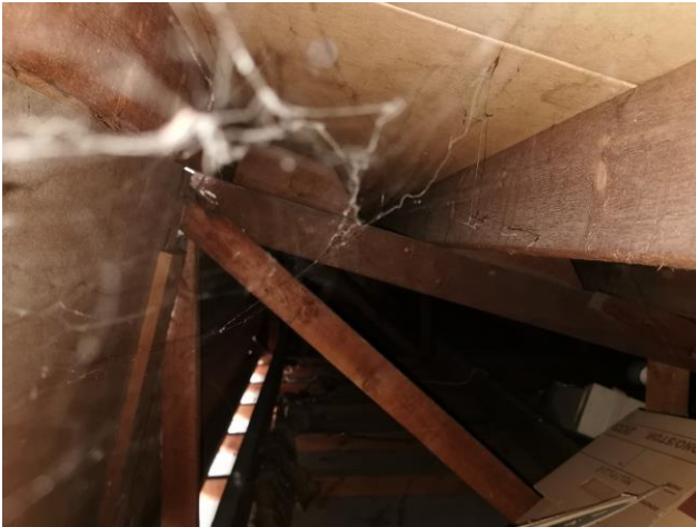
Photo 13: Roof fall loft void.
