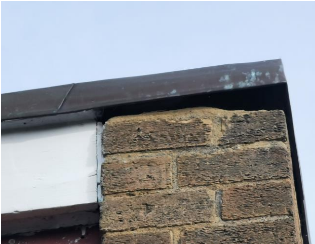
Photo 9: Gap between bricks and roof on east aspect.
