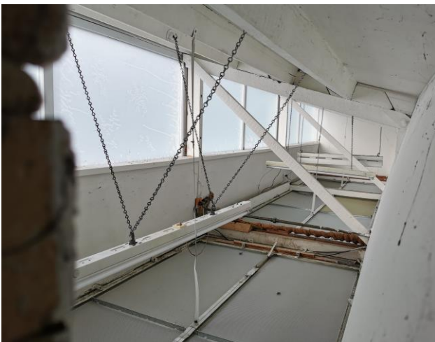
Photo 11: Roof fall loft void with windows.
