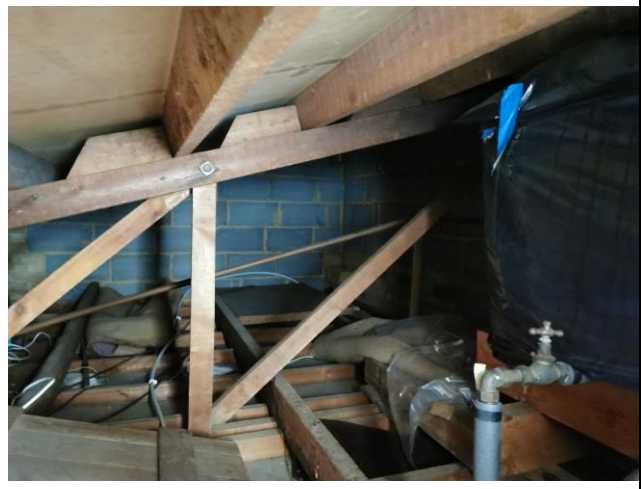
Photo 12: Roof fall loft void.
