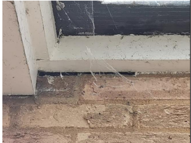
Photo 10: Crack between bricks and roof on east aspect.
