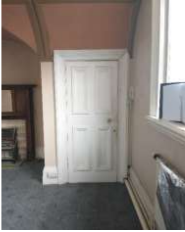
4.8 The door to Room 4 has dropped to the LHS hinge side
