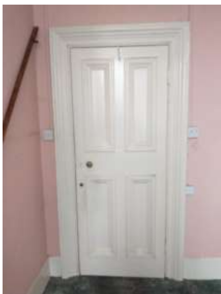
4.7 The door to Room 3 is twisted to the top of the closing door side (Left)
