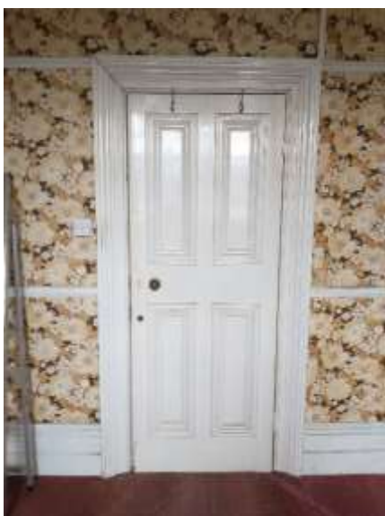
4.6 The door to Room 1 has a gap of 10 mm to the closing side, without any movement on the architrave. This is very unusual for Edwardian workmanship.
