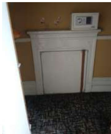
4.9 Room 1 Fireplace has been covered, this needs to be removed and the original interior hearth shown if it is still there.
