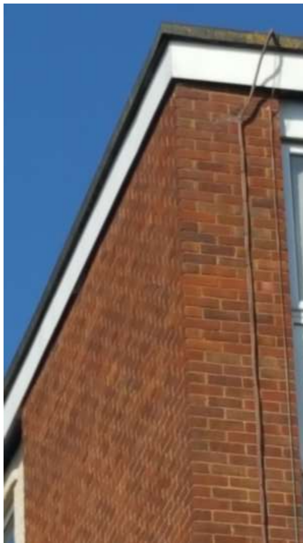
Plate 4.11 Gap under fascia on five storey residential block
