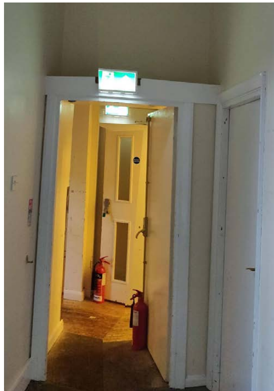
Figure 7 - The first fire exit door where we wish to remove modern fabric and adjust the position of the non-original opening.
