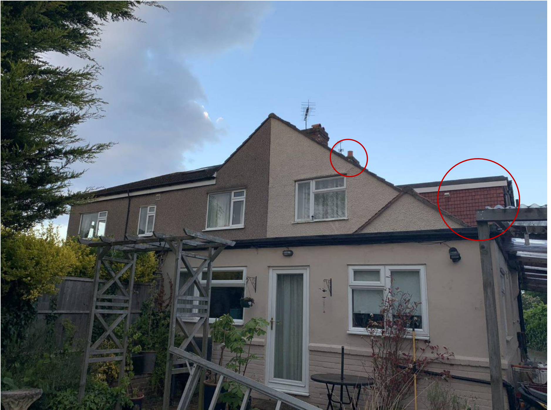
Photograph 4: Vantage point of surveyor 4 (TQ 13347 73832). Lifted lead flashing around chimney and pantiles as highlighted in the Preliminary Bat Roost Assessment were flagged prior to survey.
