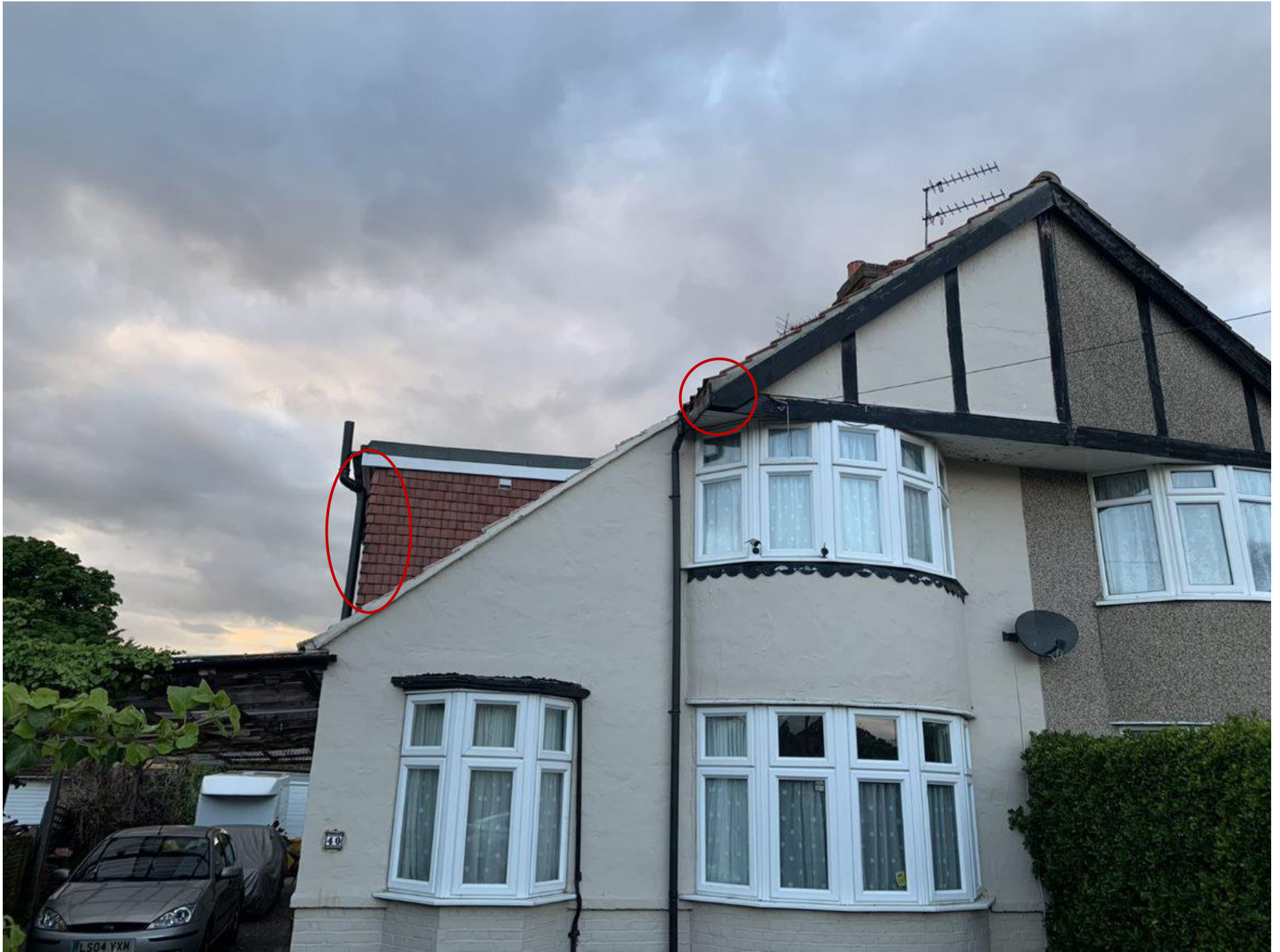
Photograph 3: South-west corner of the site, covered by surveyor 3, largely focused on the horizontal tiles. Gaps in eaves and pantiles highlighted during the Preliminary Bat Roost Assessment.
