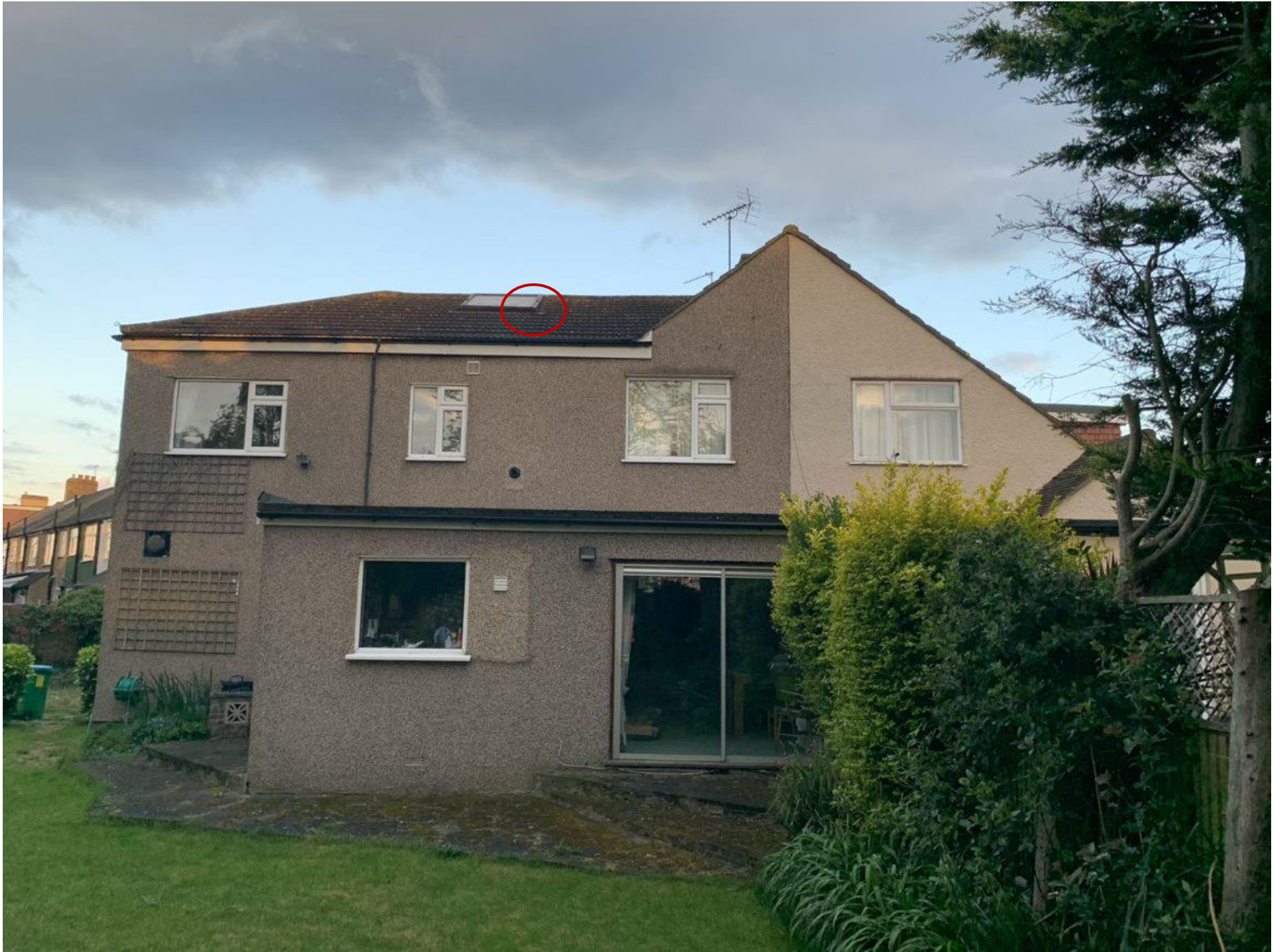
Photograph 2: Vantage point of surveyor 2 (TQ 13361 73840). Single slipped tile near Velux window highlighted prior to survey.
