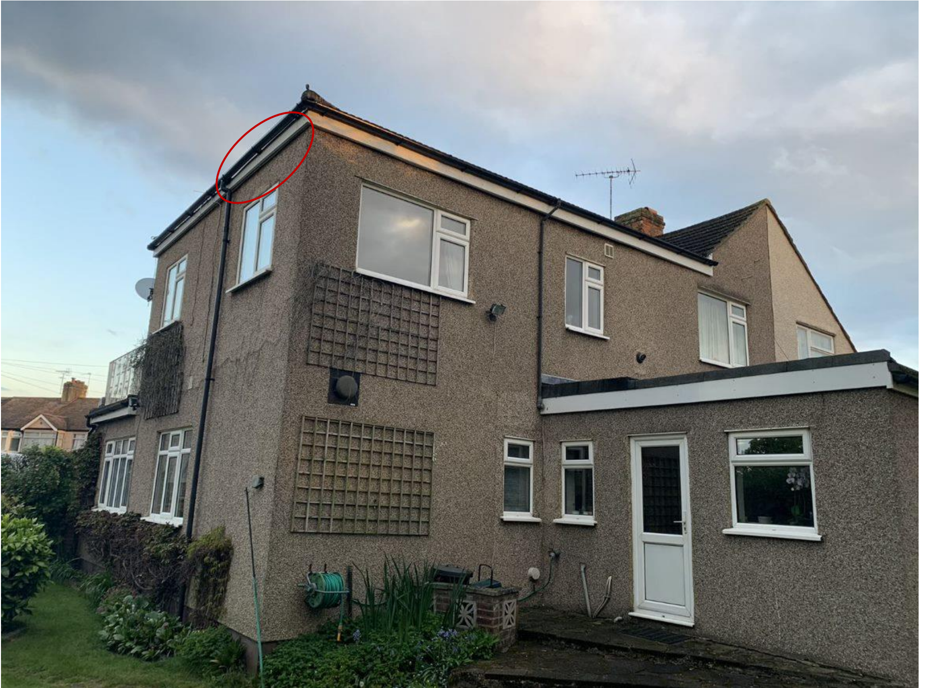
Photograph 1: East of Site – covered by a combination of surveyor 1 and 2 (Figure 2 for vantage points). Small gap highlighted within the eave, opportunistic roosting potential only.
