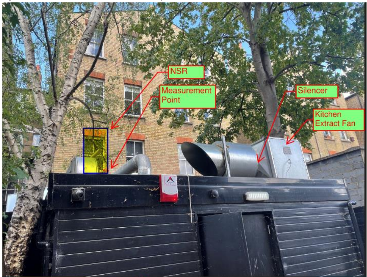
Figure 2 . Extractor fan duct, measurement position and nearest residential window
