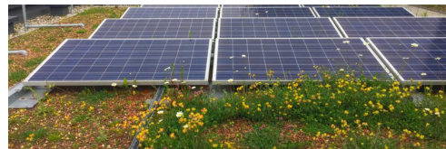
Fig. 3 & 4 PV Panels mounted on green flat roof
