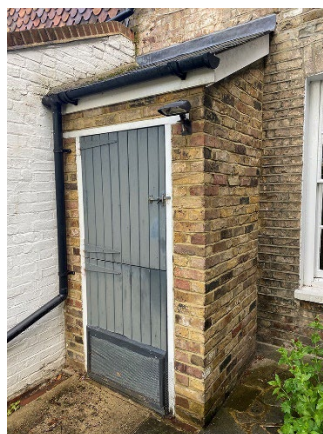
Right hand side addition showing poor brickwork not aligning or stitched into original building. Signs of structural movement above it – in connection with brickwork main extension. Poor weathering details.
