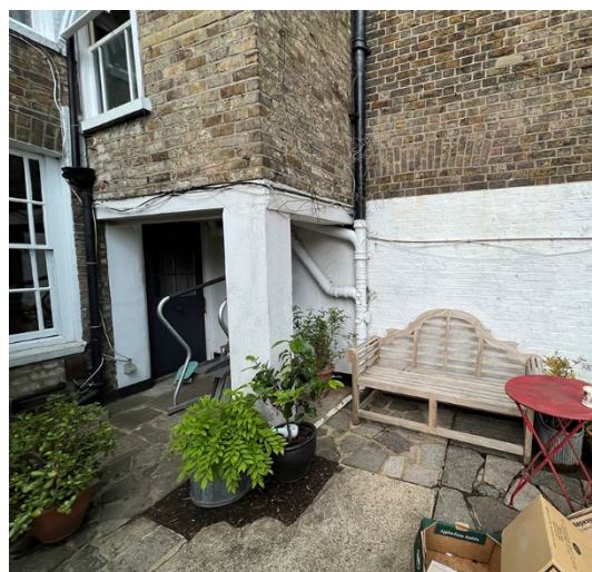
Oversized concrete pier out of keeping. Height of extension creates very low back entrance area, out of keeping with Georgian proportion.
