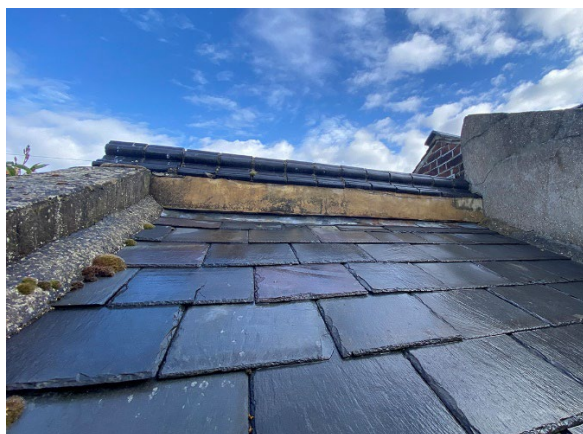
Roof of left hand side addition showing poor 'ad-hoc' detailing of 3 separate ridges finished in mixture of non-original materials, all at different levels.
