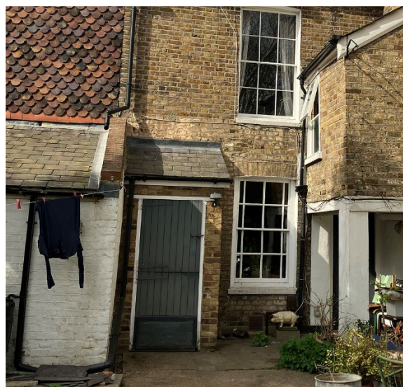
Paintwork to be removed from original rear return wall at ground floor.
