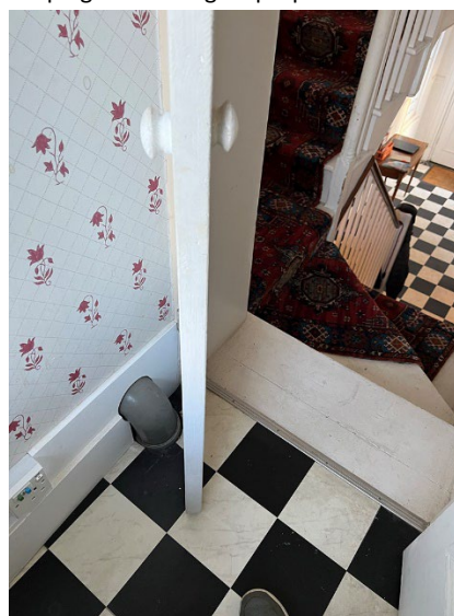
Exposed soil pipe in WC to be removed and re-routed as indicated in proposal drawings.
