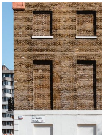
Typical 'Blind Windows' – showing set back in brickwork to add detail to the elevation.
