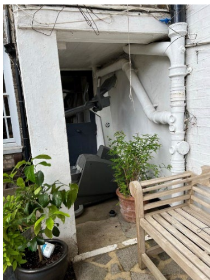
Messy soil pipes are ugly and detrimental to the original Georgian rear extension.
