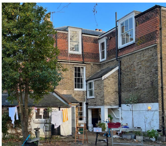
Georgian Rear elevation showing poorly placed WC 1 st floor half landing height, clashing with original windows.
