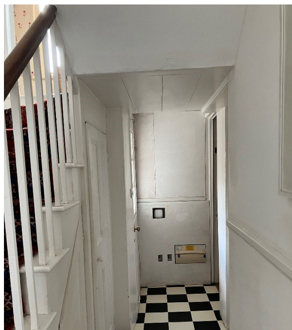
Modern Partition to be removed – as seen from hallway – also incorporates unsightly consumer unit – to be relocated)
