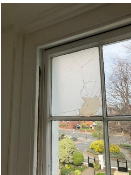
Broken window to be repaired.
