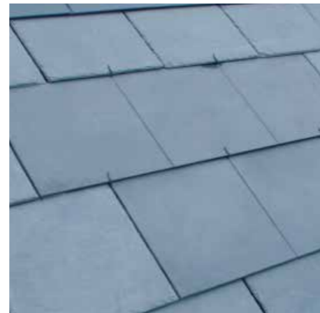
PV Slate style roofing - Units 1 & 2
